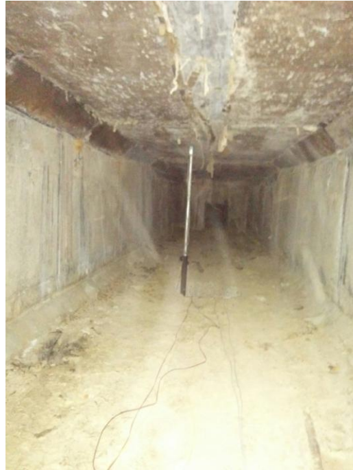
Fig 5.1 – Sensor inside Girder
