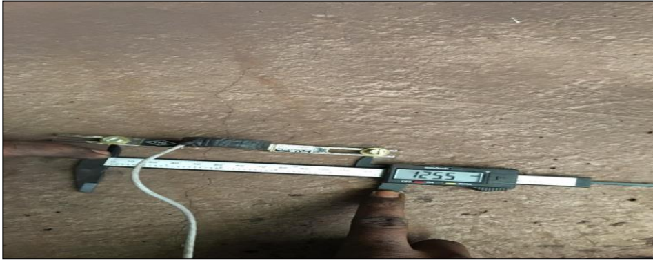
Fig 4 :- Omega Sensor and Vernier Calliper to measure crack width.
